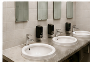
Public / Restroom Sinks
